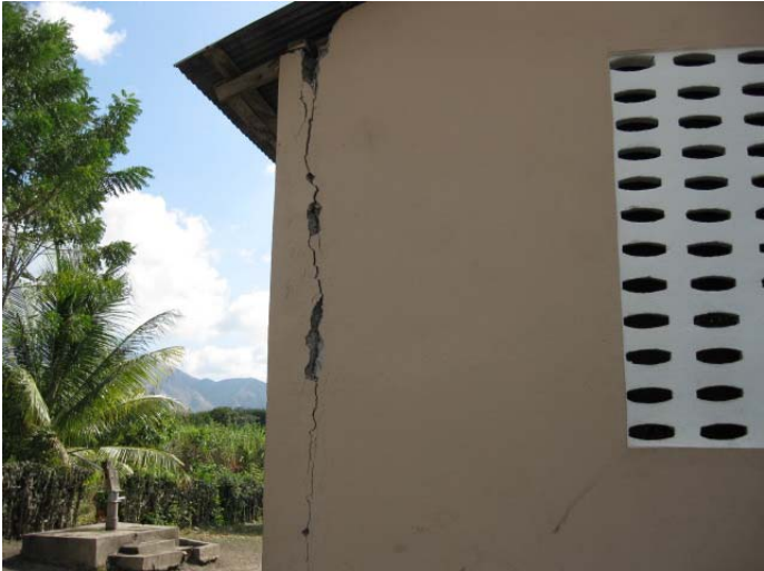
Same crack from inside church
