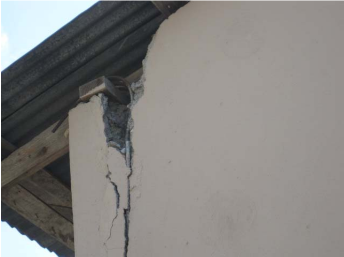
Same crack --church in Pewou
